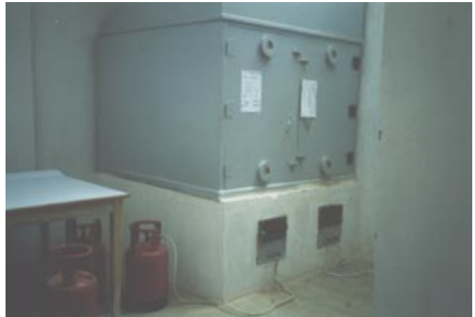
CEAS propane gas dryer in the Vonona Village
